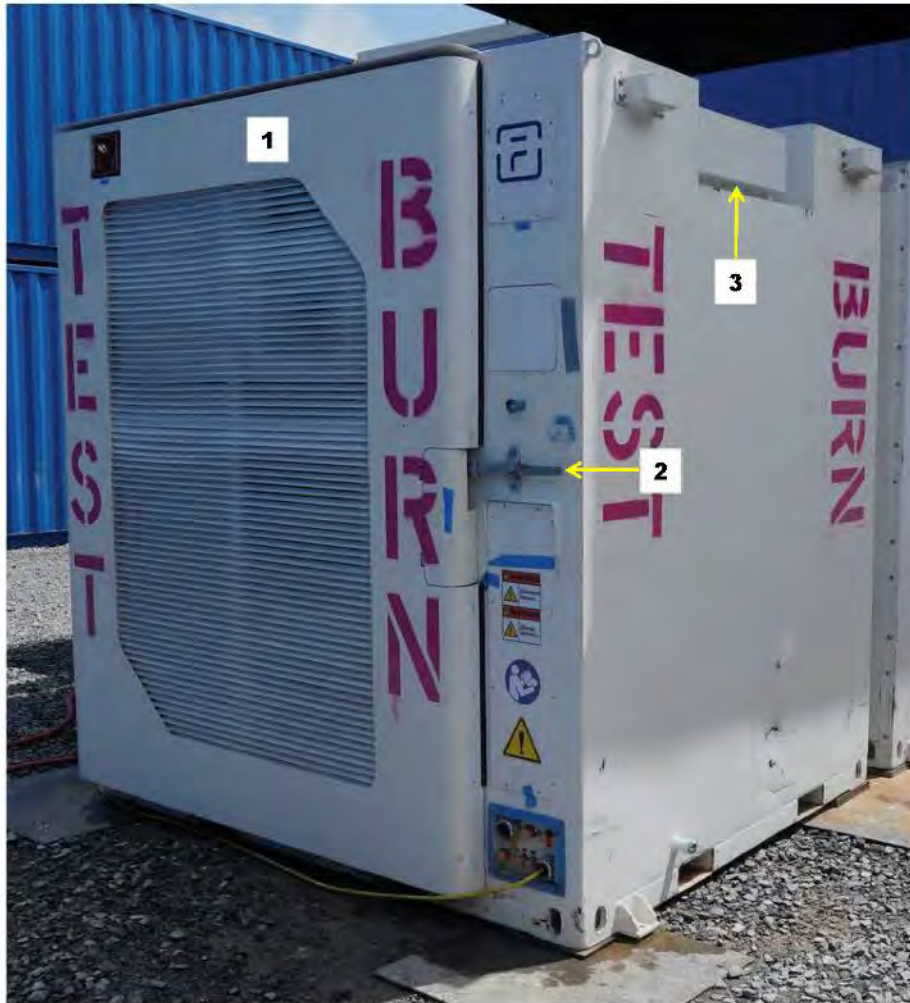
Figure 1. A photograph of a Fluence Cube.
