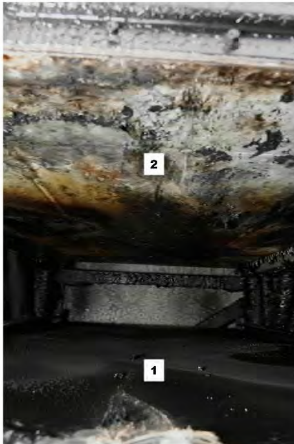
Figure 58. A photograph inside the rack after the initiating module was removed.
